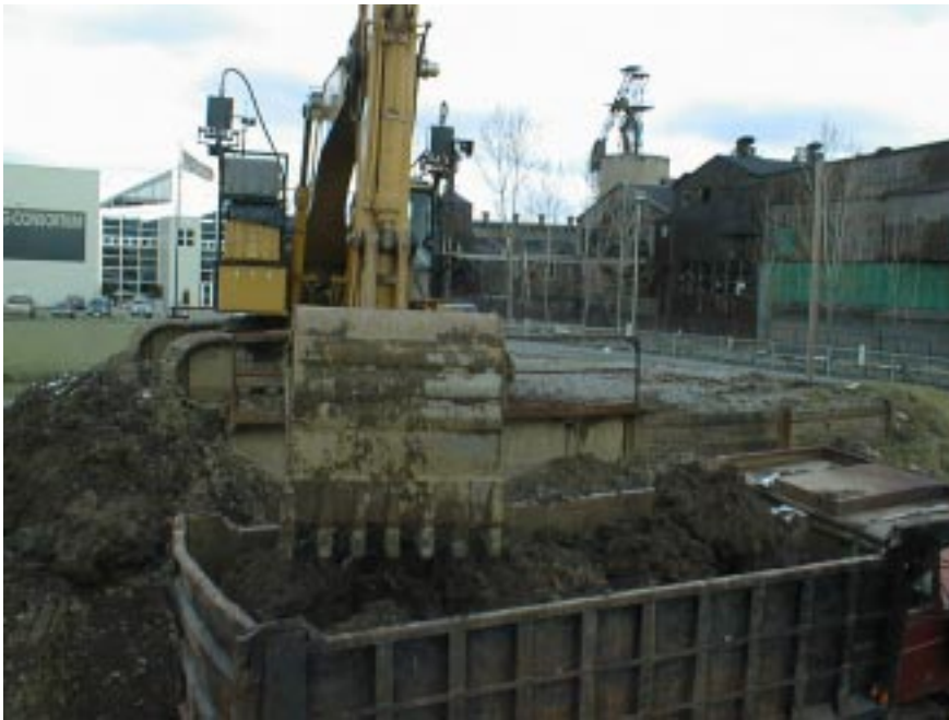
Figure 2: CMU’s computer-controlled excavator uses a pair of scanning laser rangefinders (black boxes) to recognize the truck, detect obstacles, monitor the dig face, and monitor soil in the truck bed.
